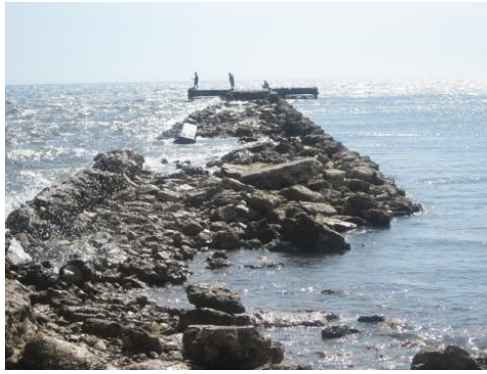
Wharf damaged by tidal wave action, coastal Rigo
