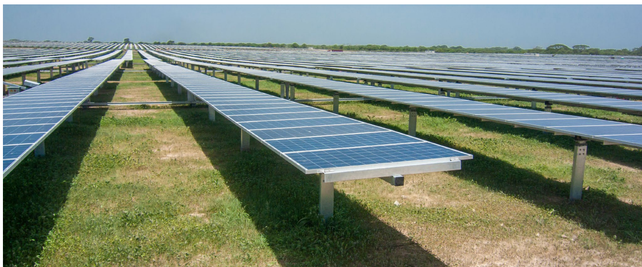
A solar power plant in Honduras
