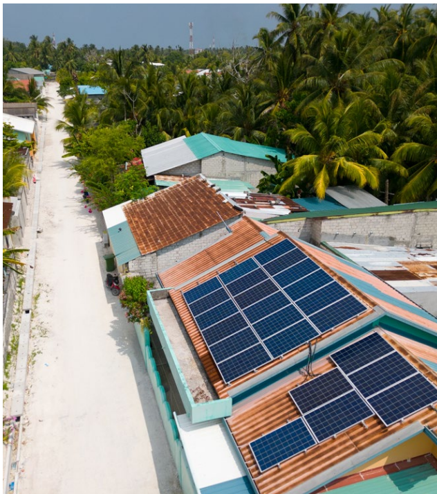
Solar panels in the Maldives
