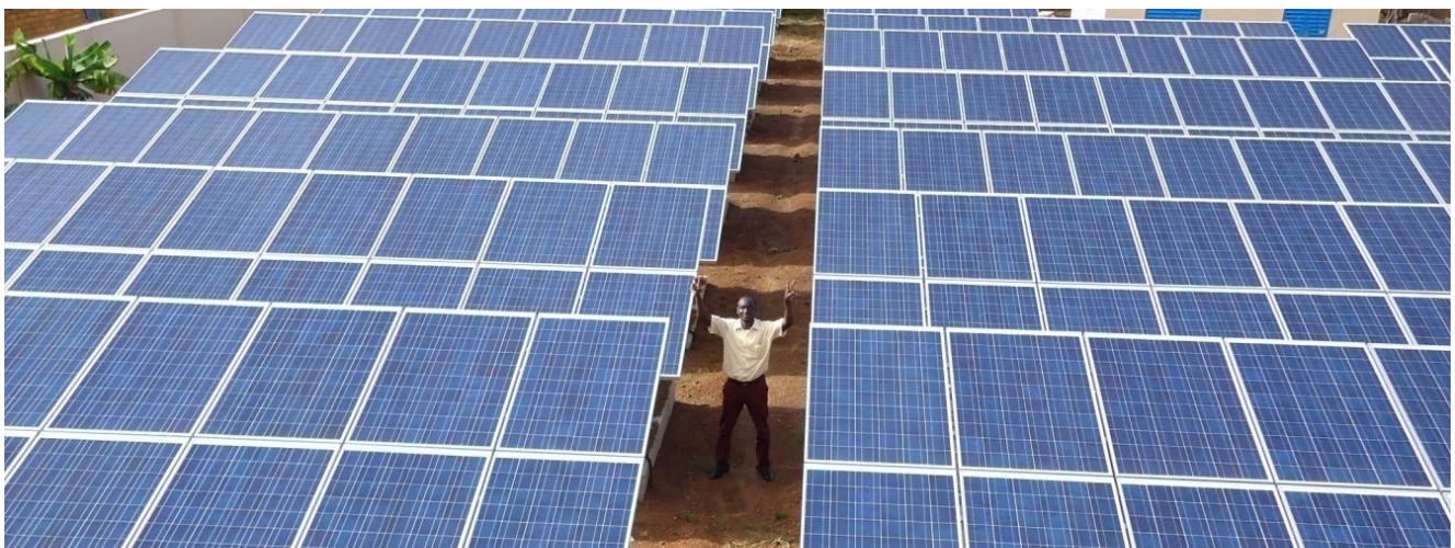
Solar facility in Kolondiéba, Mali
