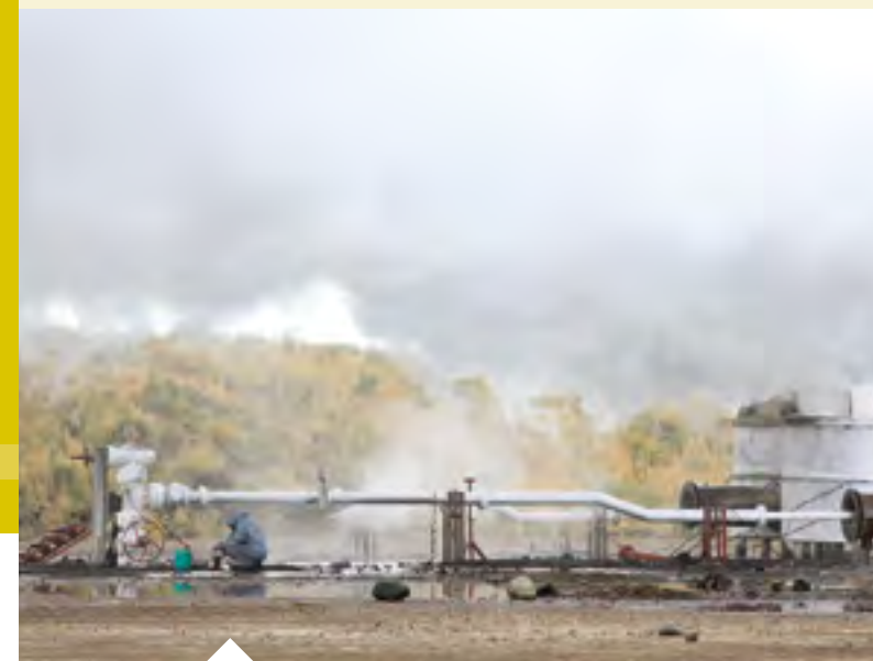
$25 million from the SREP managed by the AfDB is helping to finance Kenya's Menengai geothermal power project, which is structured as a PPP and aims to produce electricity for 500,000 households and displace 2 million tons of CO 2 emissions annually. Photo: Africa Express
