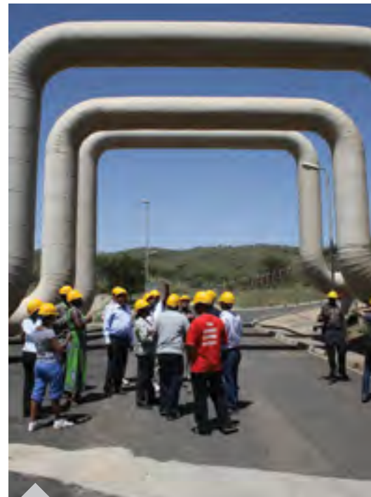
A field trip to Kenya's Olkaria geothermal power plant during the March 2012 SREP pilot countries meeting offered a first-hand look at the technology and sparked discussion. Photo: CIF
