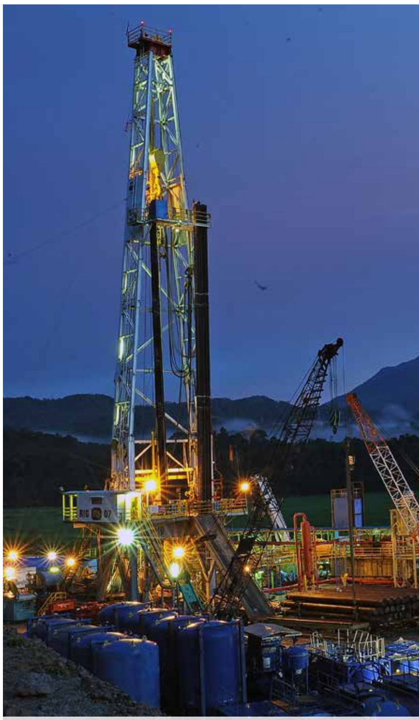
Drilling is almost complete and construction is underway at Indonesia's Ulubelu and Lehendong geothermal fields where expansion efforts, supported by CTF $125 million implemented by the World Bank, will lead to a 150 MW increase in total generation capacity. Close to 1 million households will benefit from cleaner, more reliable electricity and over 1 million tons of CO 2 emissions will be avoided annually.
