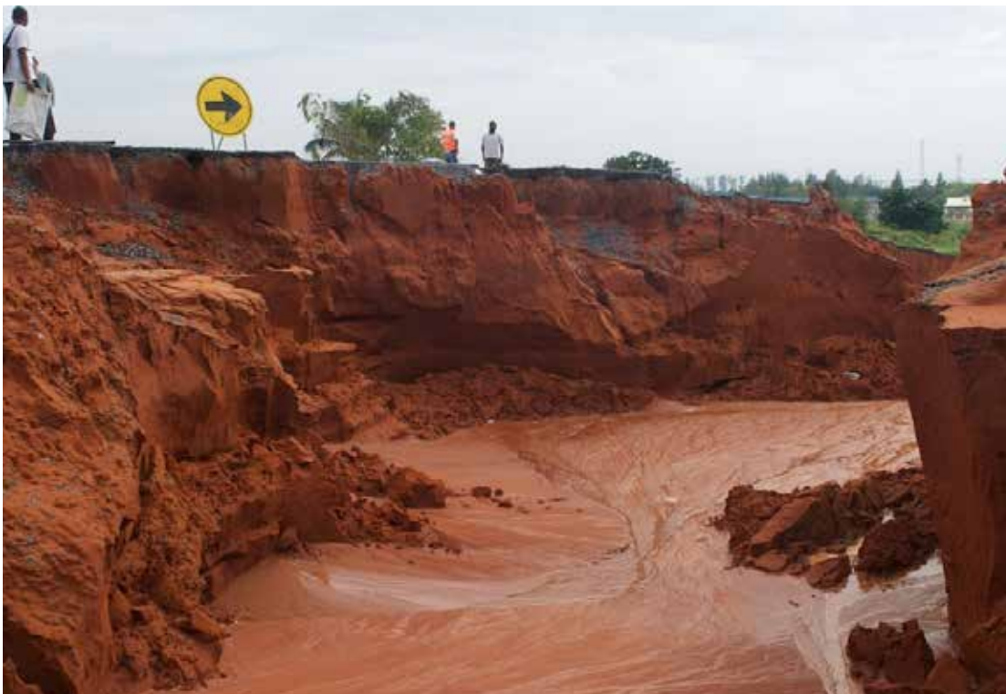
Devastating flooding in Mozambique's lower Limpopo Valley in 2013 caused an estimated $183 million in damages to the road infrastructure in Gaza province, leaving many communities inaccessible and paralyzing the transportation of goods.
