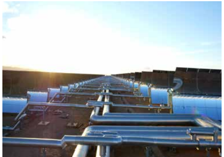
Morocco's 160 MW Noor I CSP plant (left and above).
