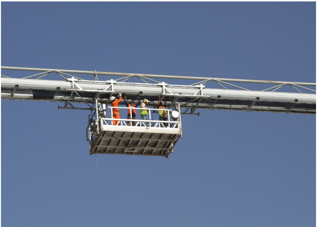
Work on transmission equipment part of a solar power plant in Rajasthan, India
